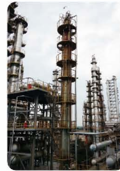
扬州石化污水汽提塔
